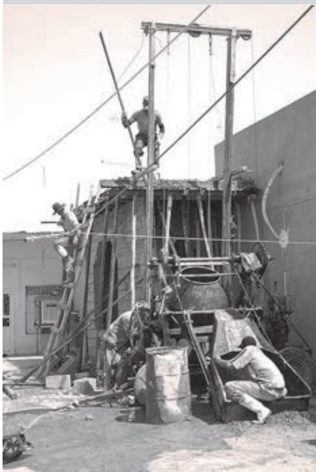
Workers repair a home damaged by a bomb blast in Taza, Iraq, in 2009. This is one of 150 homes that the UN provided funds to repair.
